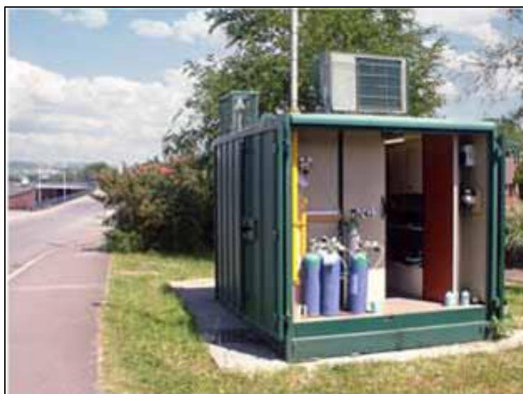
Figure 15: Automatic Urban and Rural Network (AURN) example of an automatic air quality monitoring station 363
